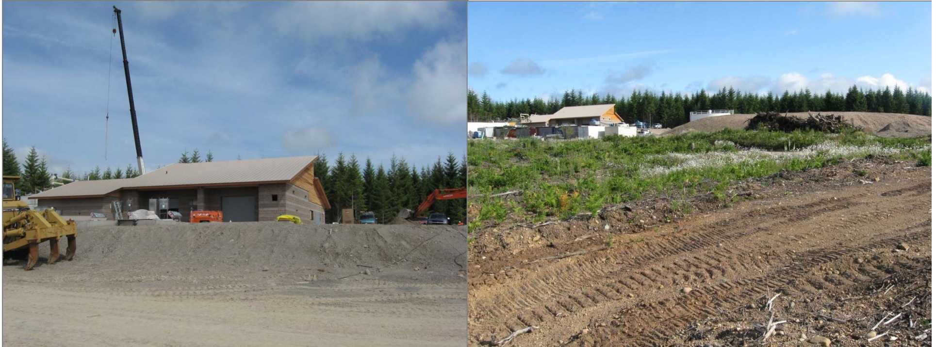
Interim Rate Ordinance Public Meeting, July 12, 2011 - Belfair Wastewater and Water Reclamation Facilities Project
