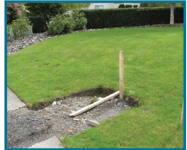
Property owners will need to build side sewers from their building to property lines, where the county utility will provide one stub, or pipe connection, per parcel.
