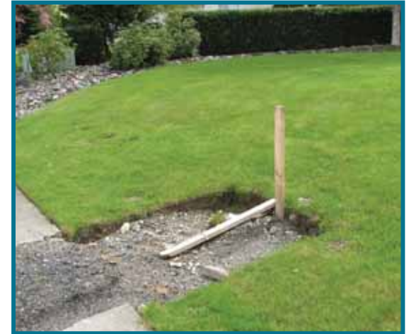
Property owners will need to build side sewers from their building to property lines, where the county utility will provide one stub (shown here), or pipe connection, per parcel.
